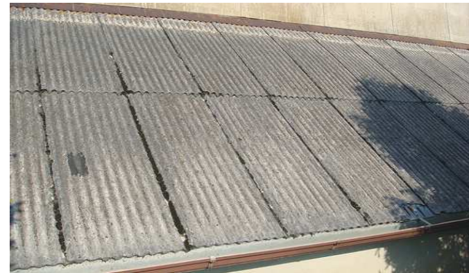
Shingles that may contain or have remnants of asbestos cement.
