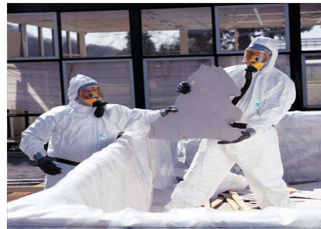
Asbestos Containing Material (ACM)
